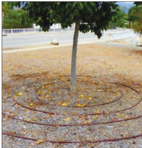
An example of a Netafim drip irrigation system in Gwinn Park. Mulch could also be added to reduce evaporation.
