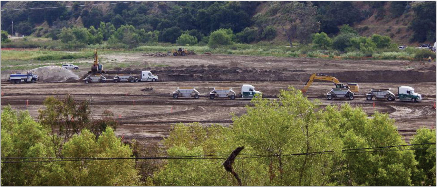
The current FCD plan would require over 400 round trips per day by heavy-duty tandem diesel trucks extending over four or more years during the dry season — presumably April through October. The trucks would enter and exit the 210 freeway via neighborhood streets adjoining the dam. The sediment would be transported to either Irwindale or Sun Valley for disposal in depleted gravel pits. Photo by Bill Christian
