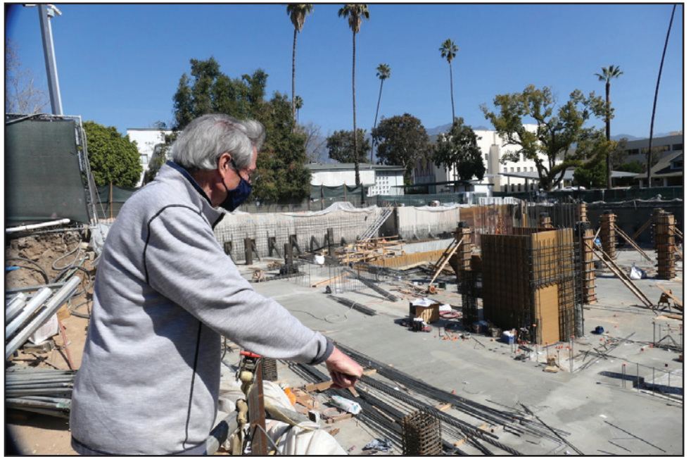
Ken overlooking construction at one of his firm's projects, The Catalonia, with 81 units at 111 N. Madison Ave., part of the Olivewood Village project in Pasadena's Playhouse Village. (photo by Avram Gold)
