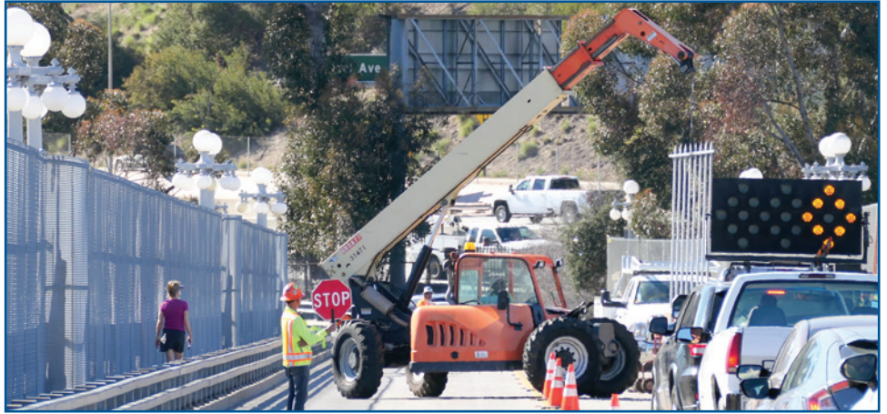
The recent scene on the Colorado Street Bridge to install mockups of the design concepts intended to discourage suicides from the bridge. (Photo by Avram Gold)
