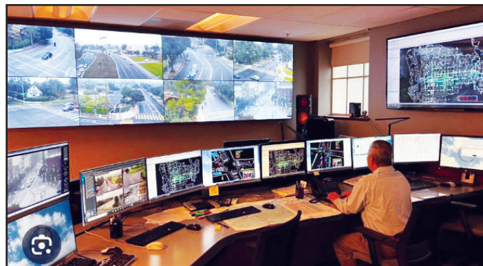
The City of Pasadena Department of Transportation operates over 340 traffic signals in its Transportation Management Center via a highly sophisticated Traffic Control System that automates and adapts to all motorized and none-motorized moving traffic occurring within city streets to maintain the traffic signal network.
