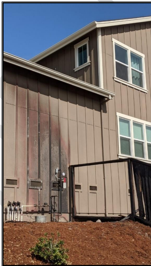
Figure 10: Home that survived the recent Glass Fire, showing impact of burning wood fence.
