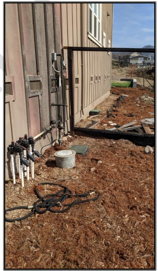
Figure 11: Same house from photo at left showing burned fence removed, and efforts by firefighters to rake away bark mulch from perimeter of home.
